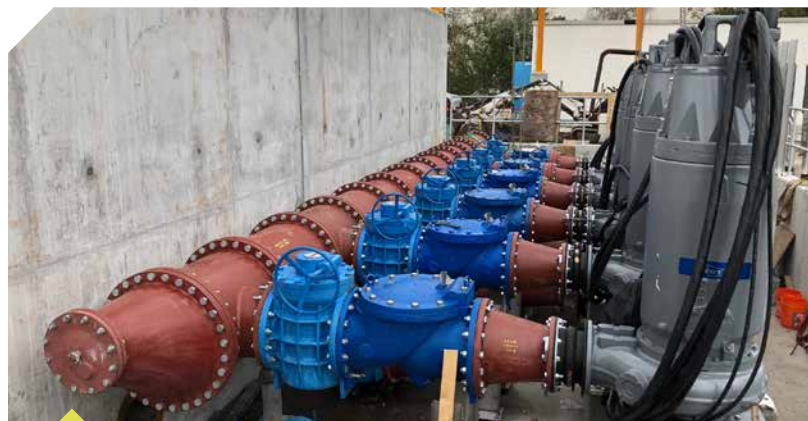
MASTER PUMP STATION PUMPING UNITS CONSISTING OF FOUR 385 HORSEPOWER (HP) MAIN PUMPS AND TWO 140 HP JOCKEY PUMPS
