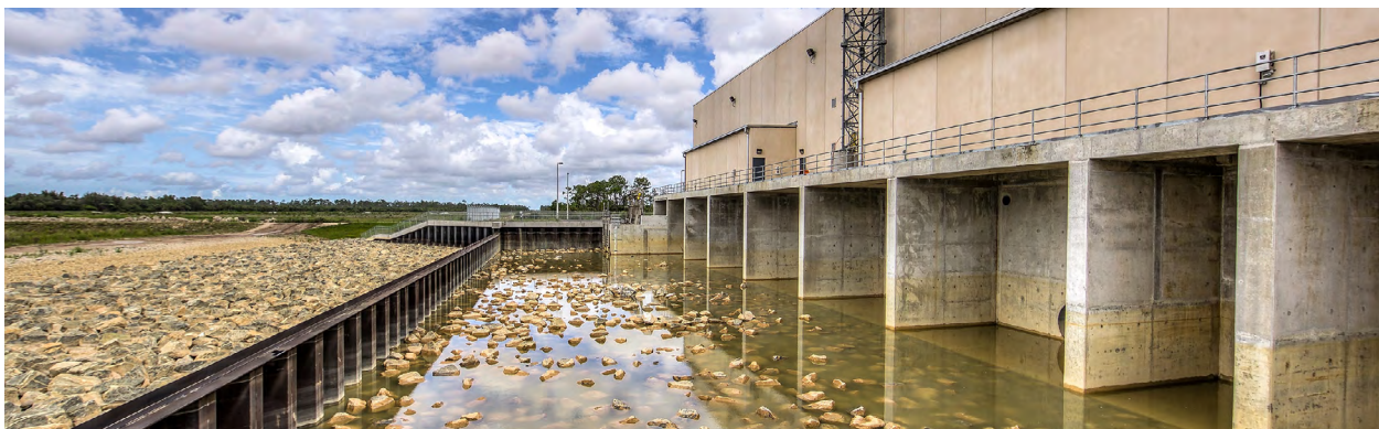
Miller Pump Station
