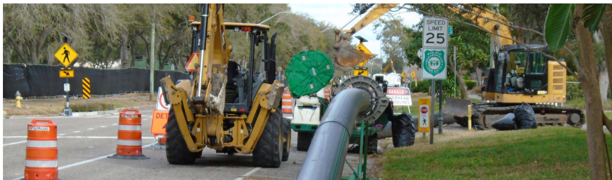
Lift Station 87, St Petersburg FL
