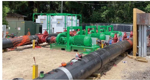
Tampa Bay Water Brandon Booster Pump Station Brandon, Florida
