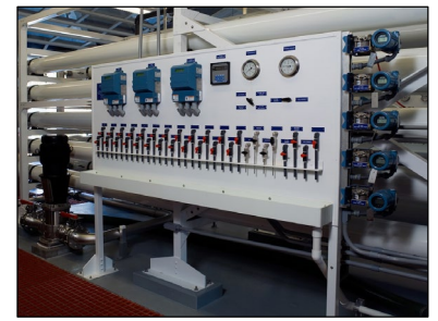
Typical RO system sampling panel allows for samples to be collected between stages for feed water, product (permeate) and reject (concentrate) streams
