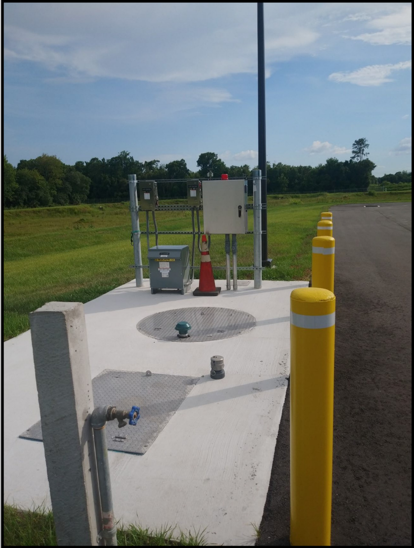
Sanitary Lift Station
