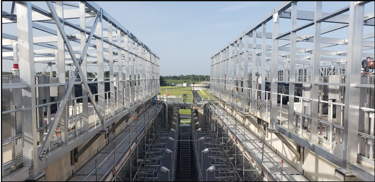
Plant 3 and 4 – Filter Cover Structure from North End Overlooking Gallery
