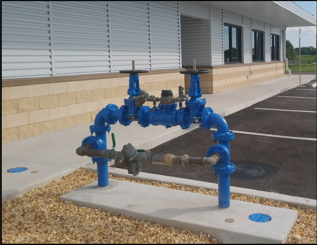
Potable Supply Connection
