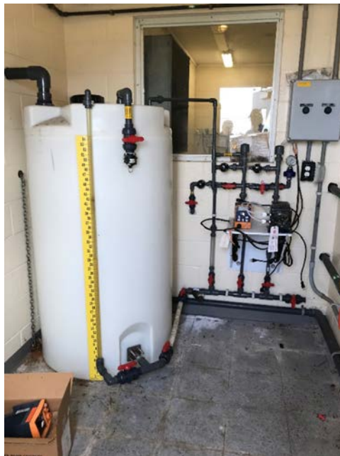
Figure 12: Liquid NH 4 OH Room
