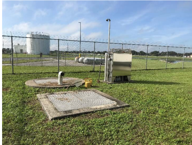
Figure 14: Wastewater Lift Station
