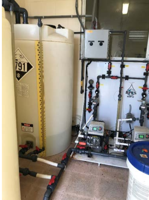
Figure 11: Liquid NaOCl Room
