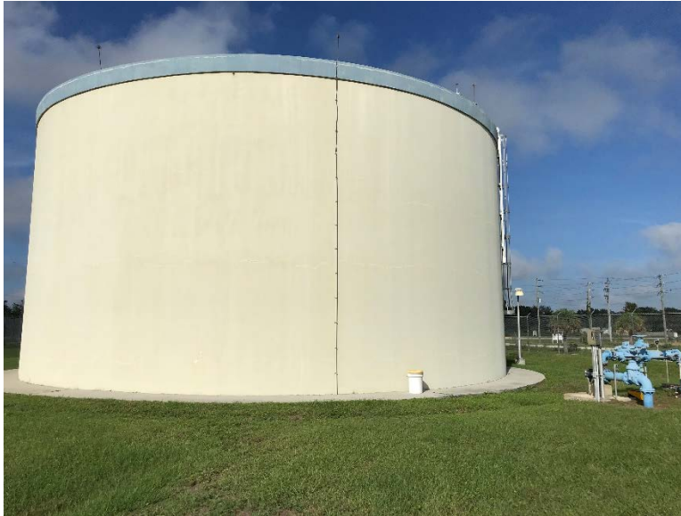
Figure 1-3: 0.5 MG Ground Storage Tank and Recirculation Piping
