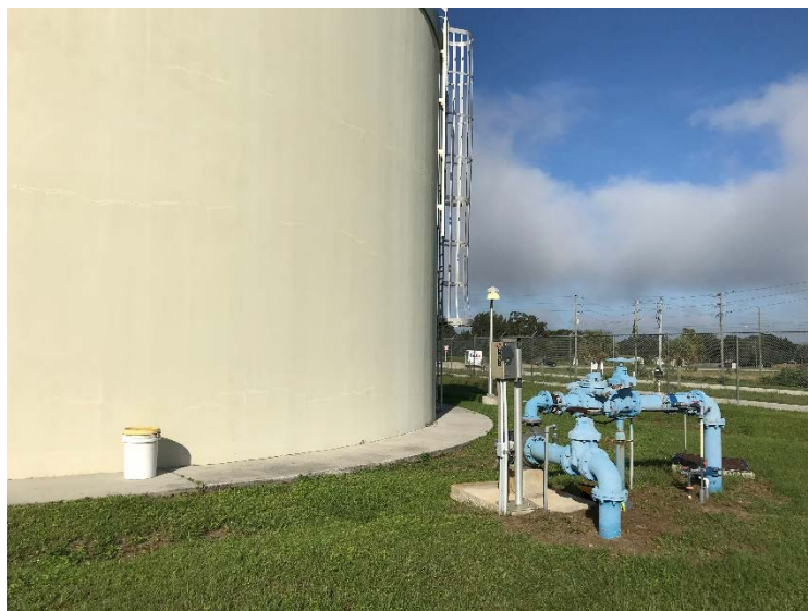
Figure 1-6: Recirculation Pump and Piping
