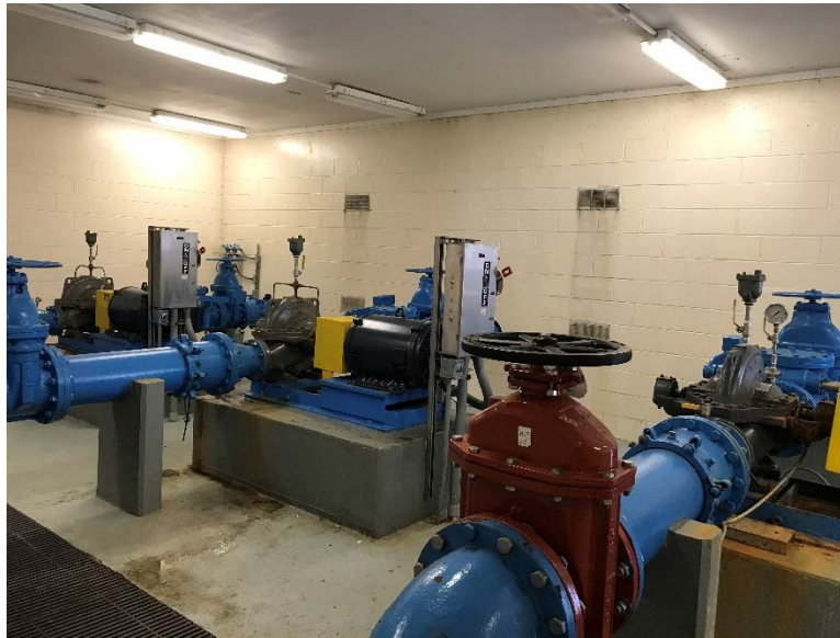
Figure 1-8: High Service Pumps
