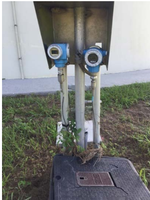
Figure 1-4: Redundant Tank Level Transmitters
