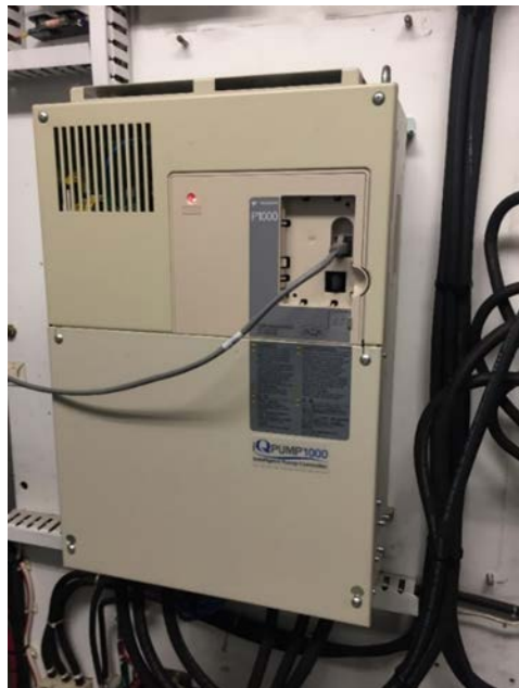
Figure 10: Variable Frequency Drives
