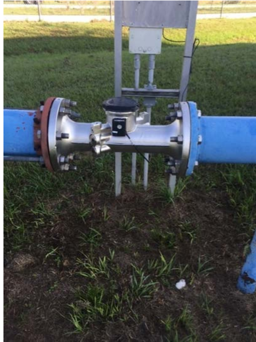
Figure 1-5: Battery Powered Octave Ultrasonic Meter (Influent)
