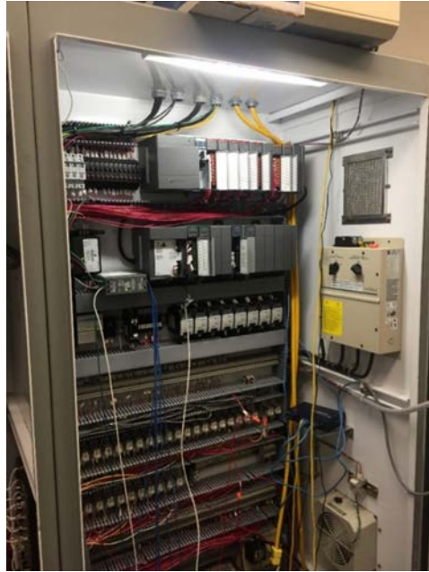
Figure 1-9: Existing PLC Control Panel
