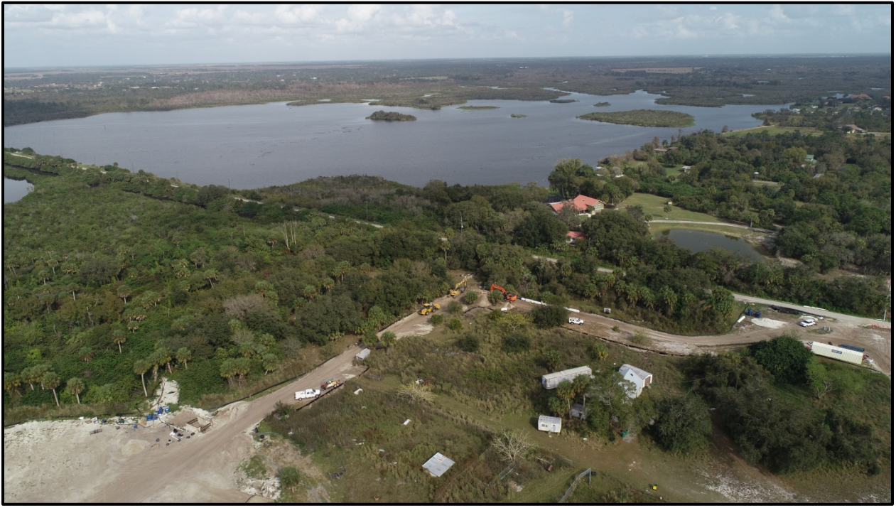
Pipe installation from south end of HDD, crossing under Shell Creek, Towards Shell Creek WTP – January 2020
