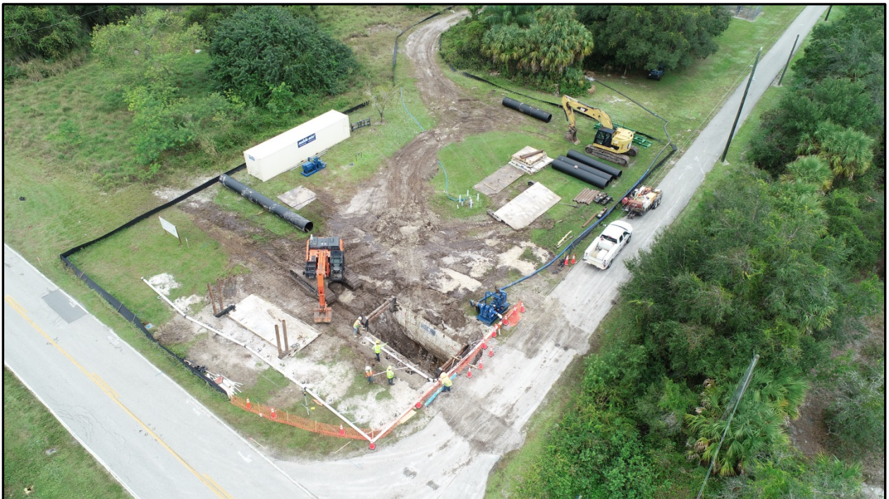
Jack and Bore Preparation at Shell Creek Reservoir, Dam Road – South Side of Shell Creek Nov. 2019
