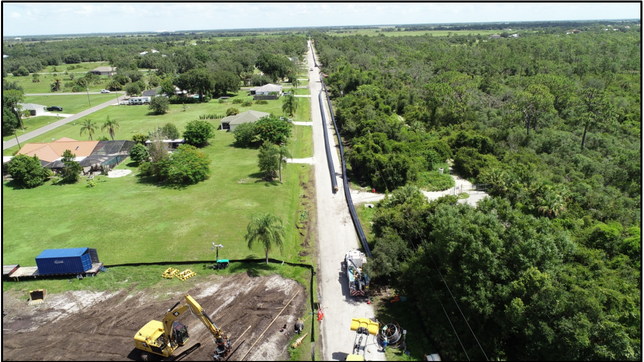
HDPE pipe fused and ready for Pullback on north side of Shell Creek, July 6, 2019
