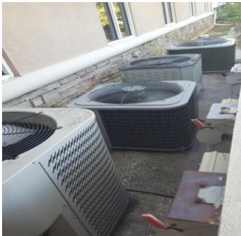
Pad-Mounted HVAC Components
