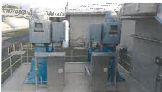
Plant #3 Finished Water Transfer Pumps (Lead and Back-up)
