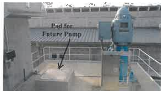
Plant #4 Finished Water Transfer Lead Pump (Lead and future back-up location)
