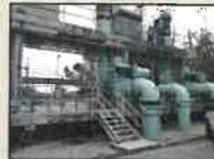
Raw Water Pumping
