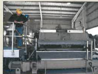
Sludge Belt Presses
