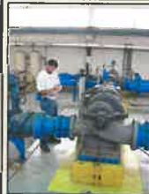
High Service Pumping
