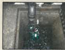
Sump Pumps/Lift Stations
